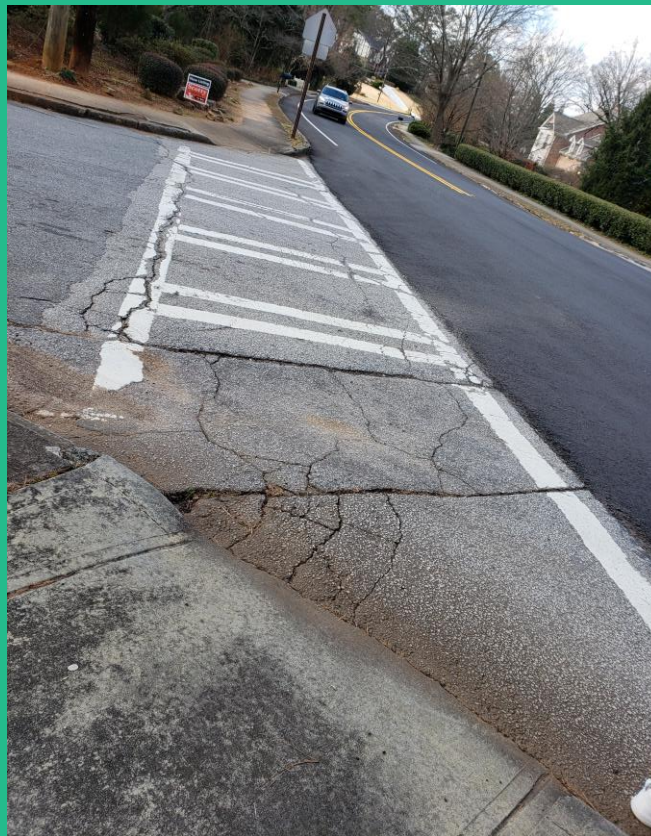
Figure 19: Damaged curb cut and pavement at intersection with Midvale Court/Crestcliff Drive
