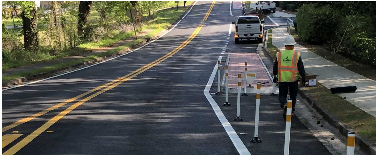
Brockett Road Traffic Calming (Source: City of Tucker)
